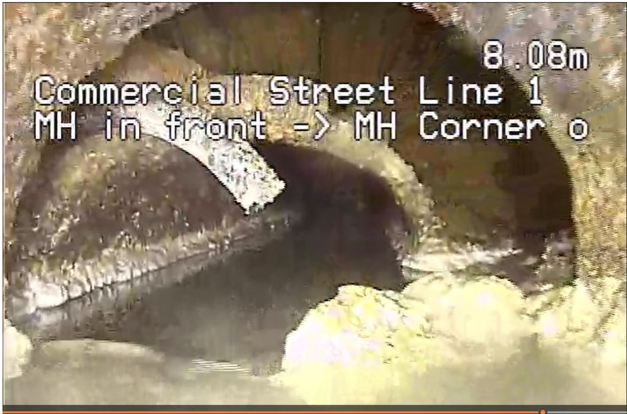
Figure 4: CCTV screen shot (Feb 2025) with the camera stationed ~8.1 m forward of the Wilson's Pharmacy northernmost driveway. Sections of the pipe are circumferentially missing.
