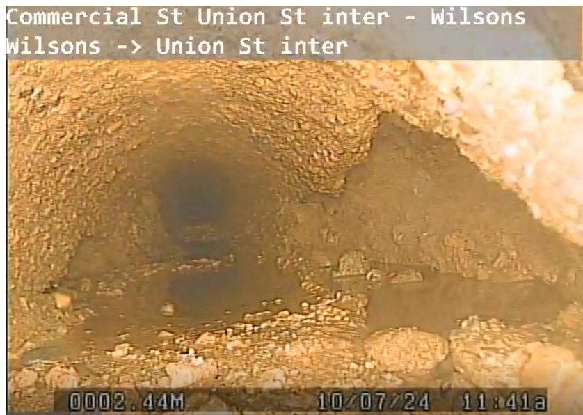
Figure 3: CCTV screen shot (Oct 2024) with the camera stationed ~2.4 m forward of the previous screen shot. Sections of the pipe are missing at the 3:00 and 9:00 quadrants of the pipe; concrete debris is visible in the water level.
