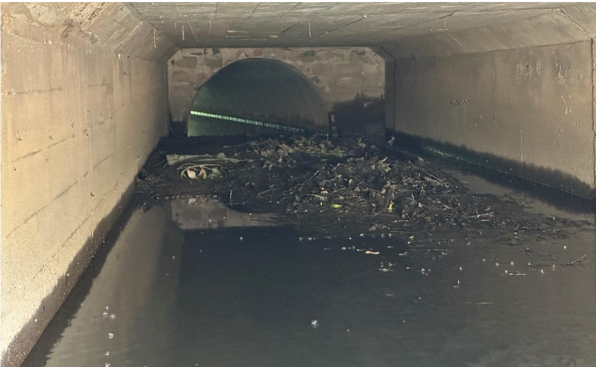
Figure 5-3: Example of Blocked Infrastructure on Commercial Street due to Sediment and Organic Matter Buildup
