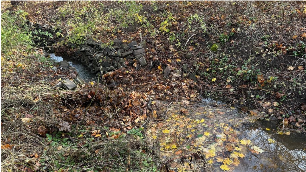
Figure 5-2: Example of Ditch Blockage in Horsburgh Drive Ditch
